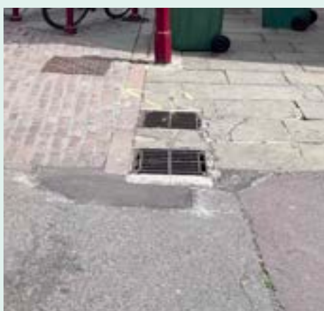
Untidy, cluttered and poorly maintained paths and roads was raised by many people. A cohesive street furniture and maintenance strategy could be key to ensuring that Newark's street remain accessible to all and in keeping with the built heritage.
