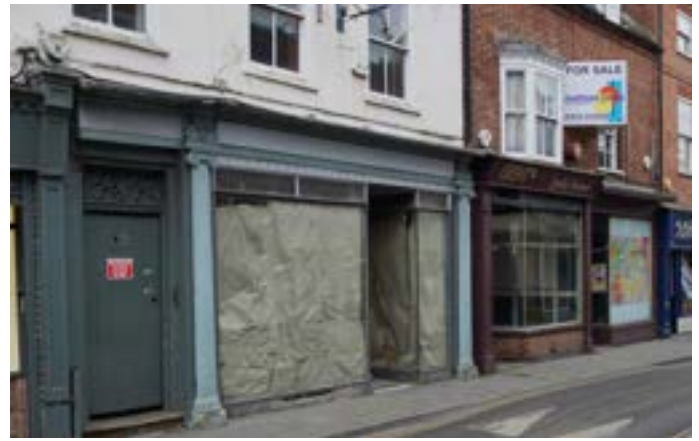
Empty shop fronts in vacant units create an untidy public realm and highlight declining retail in the centre
