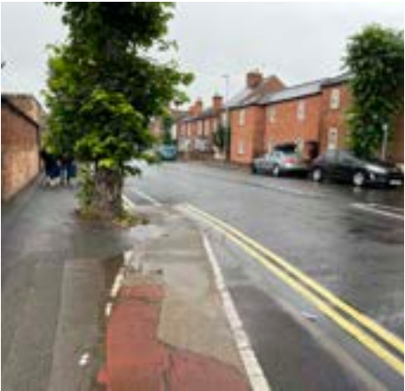
Poorly maintained cycle lanes
