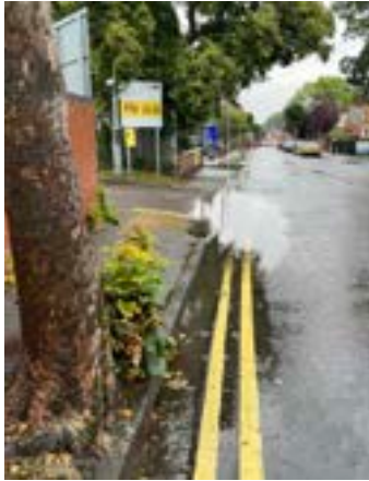
Poor drainage on Appleton Gate
