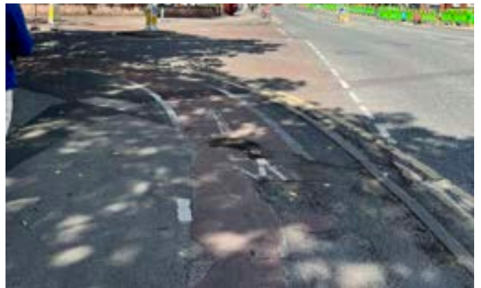
Cycle lane on junction of Appleton Gate and Queens Road is in poor condition.
