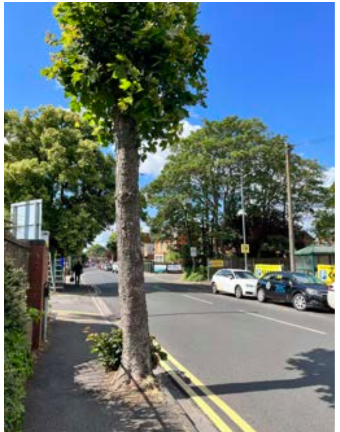
Trees up-rooting the pavement along Appleton Gate
